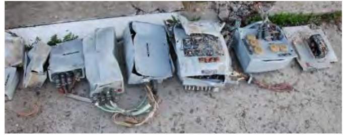
Figure 1.17: Junction and control boxes of electrical installation. Photo taken at the site of wreckage storage [16].
